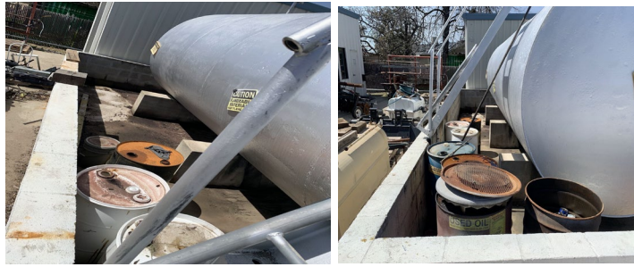
Figure 4A Image of the oil tank area showing the clutter of old oil drums.
