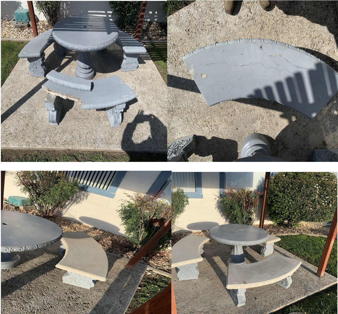
Figure 8. Before and after images of the replacement of the cracked and broken tops of the park benches.
