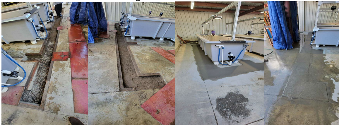
Figure 7. Before and after images of the repaired floor around the outdoor fish tank area.
