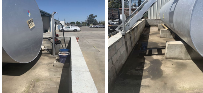
Figure 4B Image of the oil tank area after it was cleaned and decluttered.
