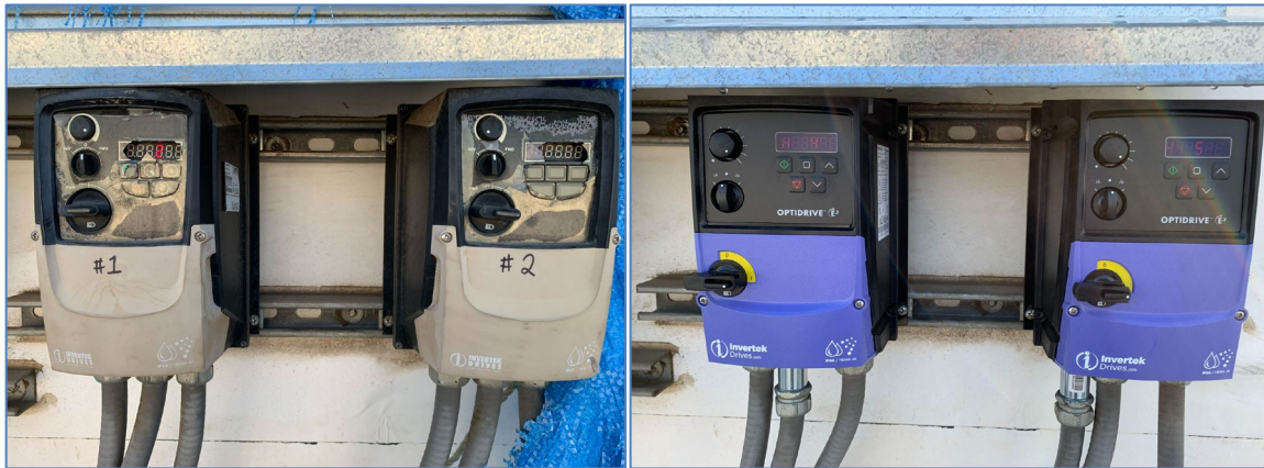
Figure 7. Old VF drives (left) and their replacements (right).
