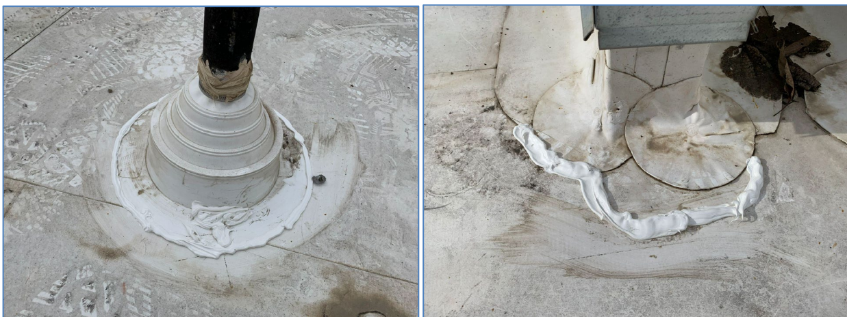
Figure 6. Temporary repairs to prevent water leaks on the roof of the fish hatchery. The TPO boot (left) was repaired and the patch seals (right) checked.
