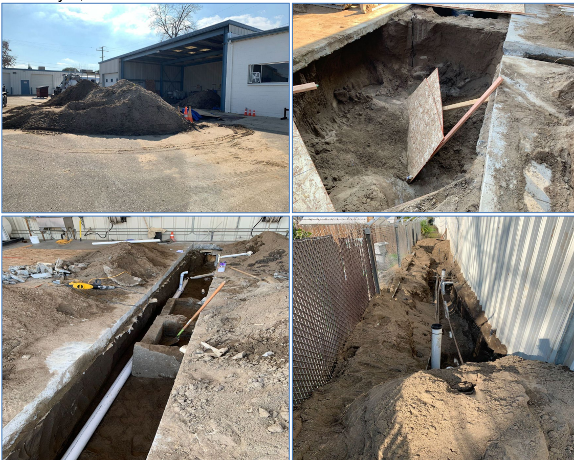
Figure 4. The DMVCD plumbing project in front of the wash bay and behind the wash bay building.
