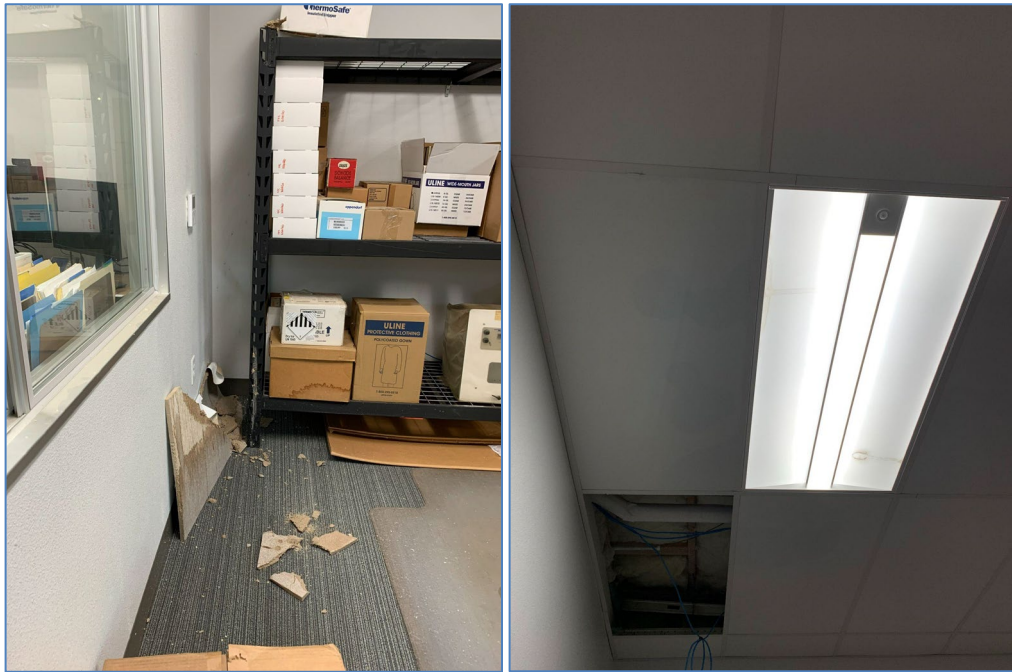
Figure 5. A water leak caused minor damage to the offices in the new fish hatchery building.
