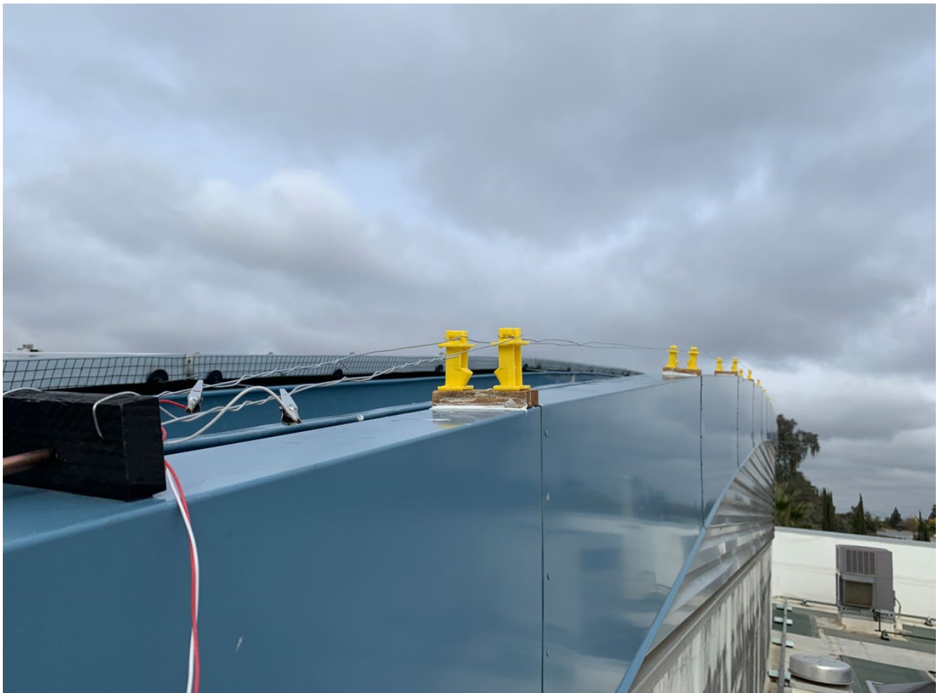
Figure 1. Bird electric wire installed to prevent bird activity.
