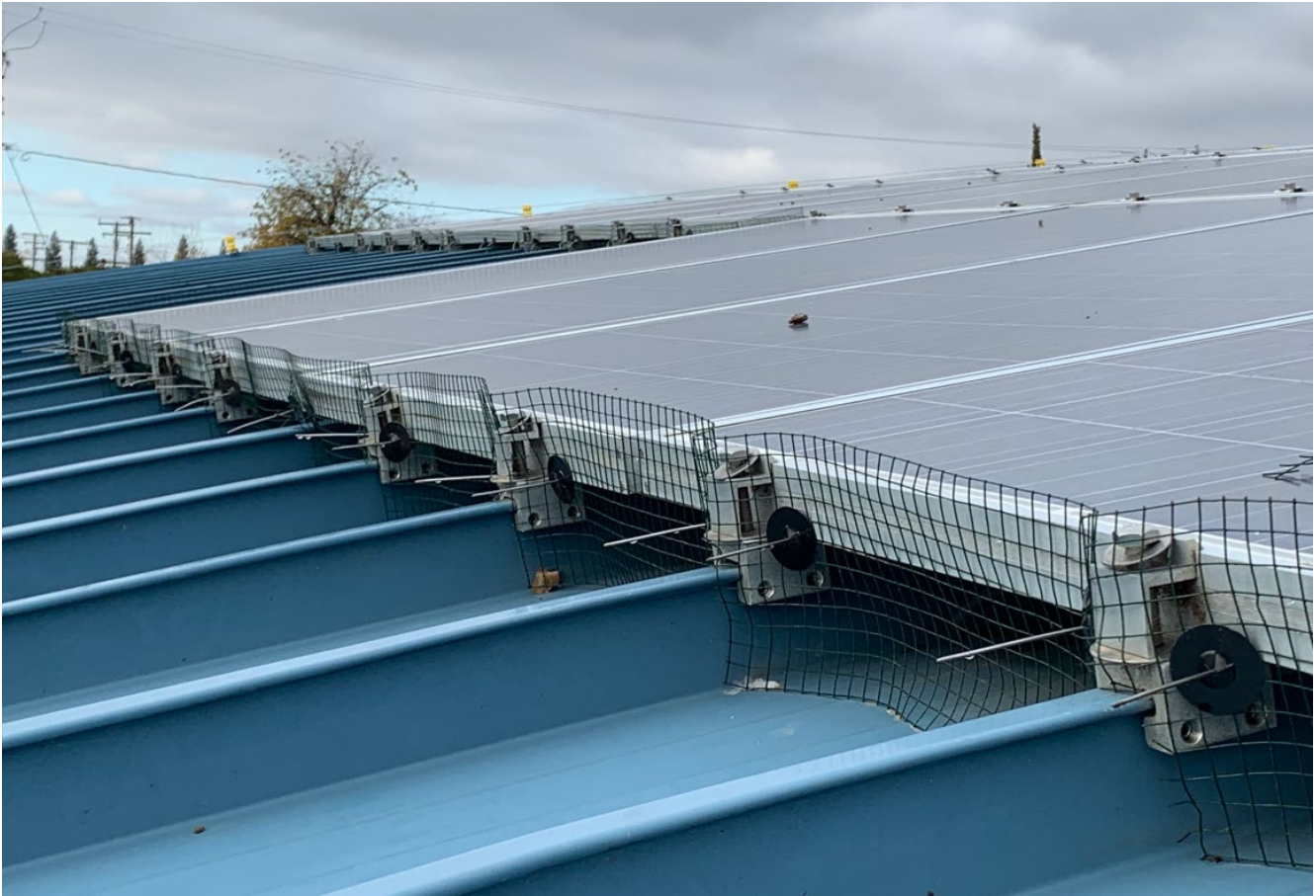
Figure 2. Bird exclusion material installed around laboratory roof solar panels.
